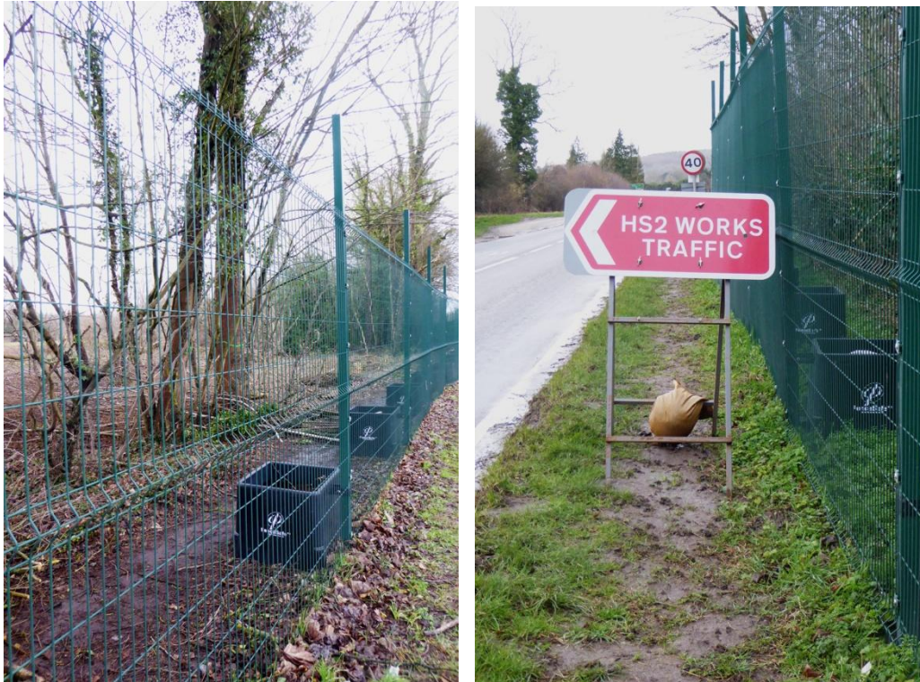
West side – the security fencing, constructed on the existing footpath; further gratuitous obstruction of the limited space remaining, by a road sign
